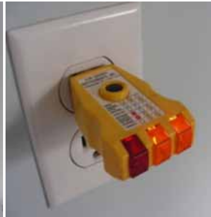
second test on same receptacle shows no problem
